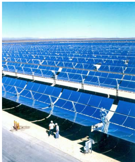
Figure 1.1: Solar thermal trough plant in Kramer Junction, California (Source: Sandia National Laboratories, Albuquerque)
